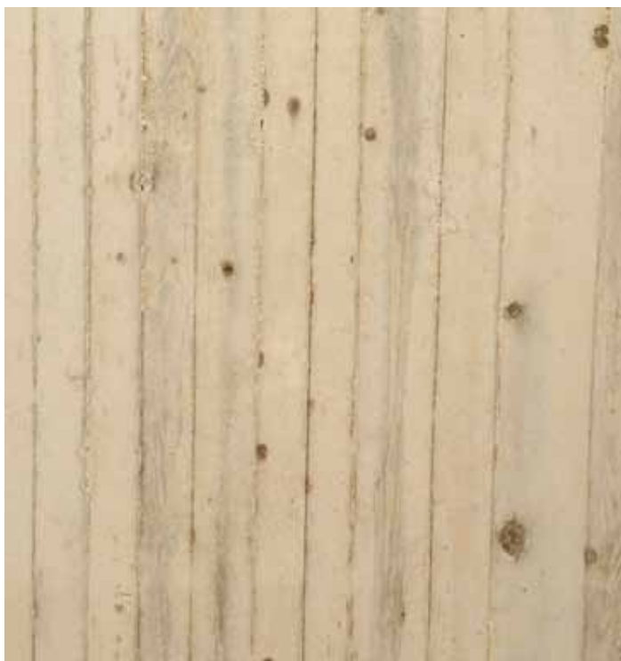
The irregularities in a concrete shutter imprint.
